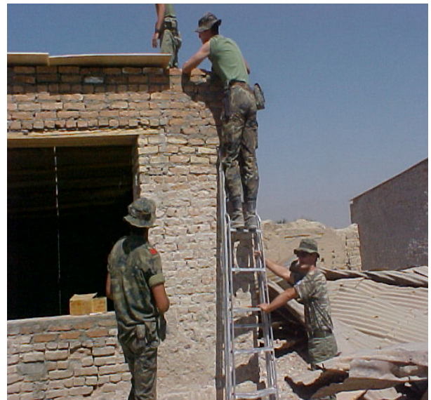
Reconstruction works in a school building in the suburbs of Kabul made by GRC NCOs_ July 2002
